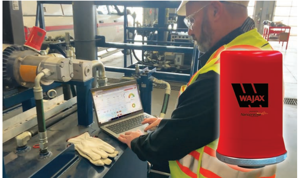
TechIQ condition monitoring sensors (inset, right, and left on motor) leverage wireless connectivity to enable real-time monitoring, early fault detection, and predictive maintenance.
